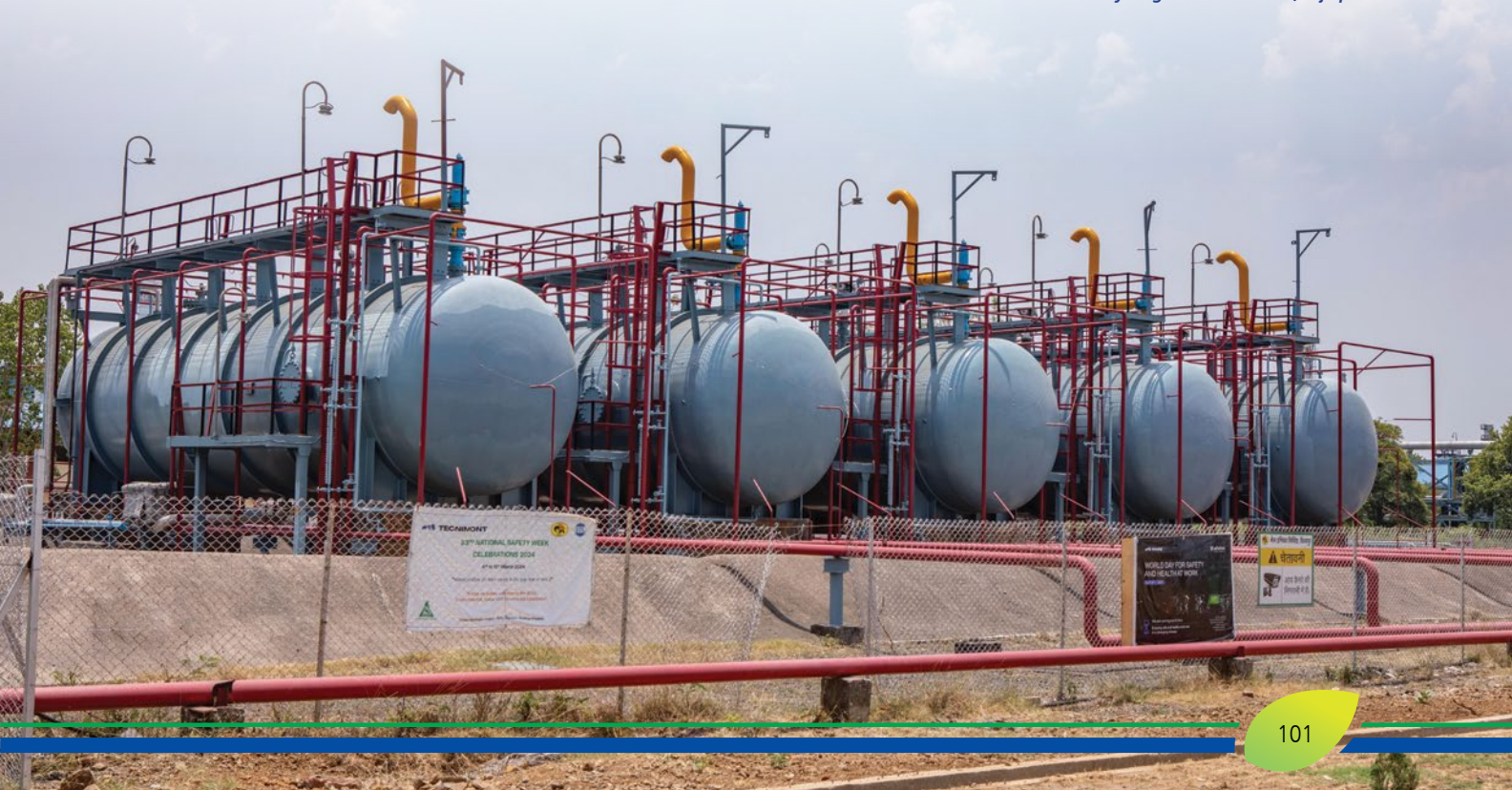
10 MW Green Hydrogen Plant in GAIL, Vijaiapur
