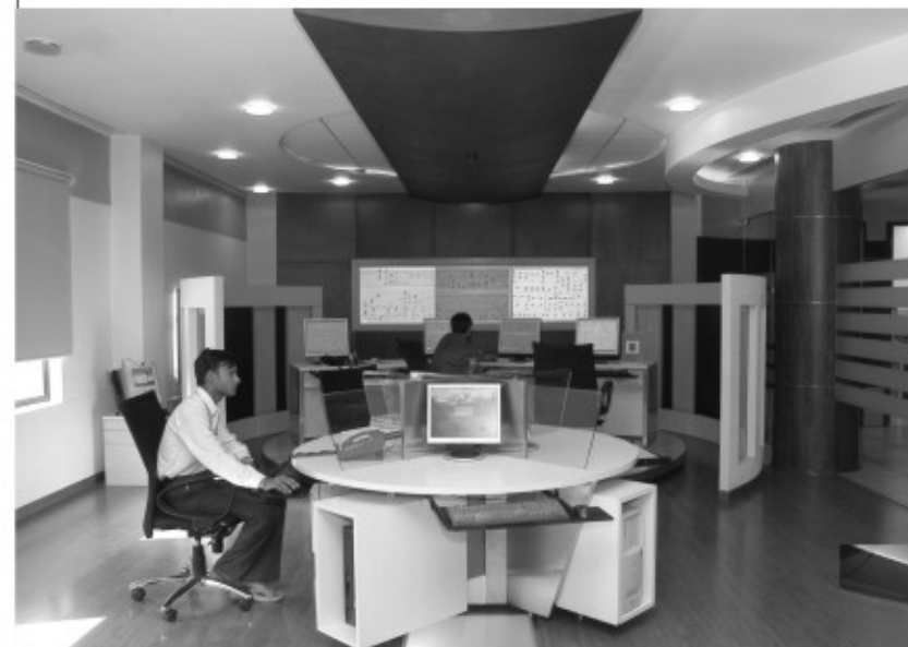
IT Infrastructure at GAIL
