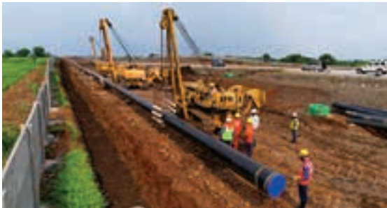
Laying of Natural Gas pipeline from Mumbai to Nagpur under MNGPL project
