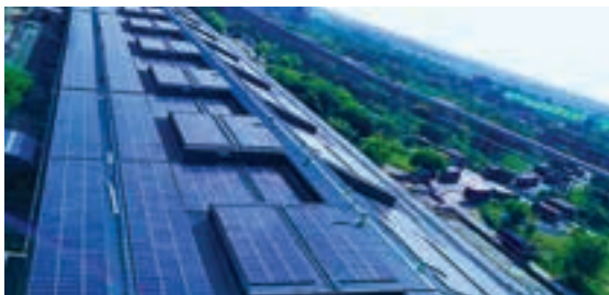
Roof top Solar Project at GAIL, Pata Petrochemical Plant
