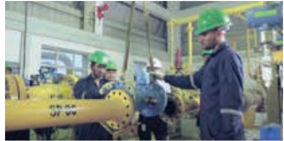
Meter Prover Facility at GAIL, Hazira
