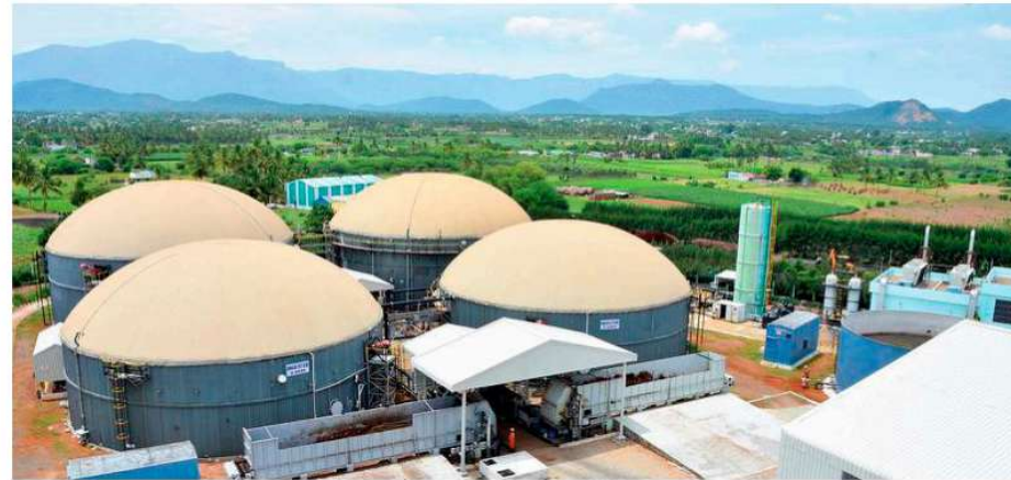
GREEN FEEDSTOCK. Compressed biogas plants are set up in rural areas for assured supply of biomass
