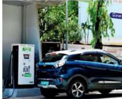
Electric vehicle charging facility at an IndianOil fuel station
