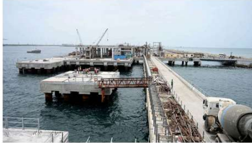
ENHANCING CAPACITY. The jetty will add 3 million tonnes of cargo per annum to the port's capacity BUJOY GHOSH
