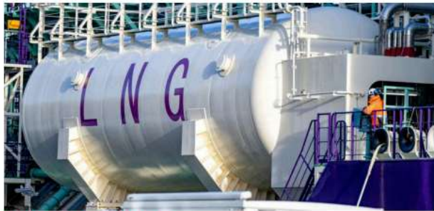
CHALLENGES AHEAD. Indian demand for LNG cargo in the spot market is expected to slow down over the next two years
